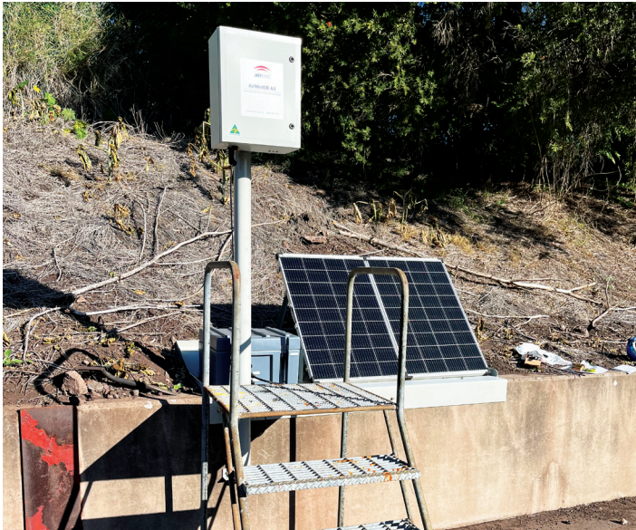
One of the 5 new Koppers air monitors around our boundaries.
